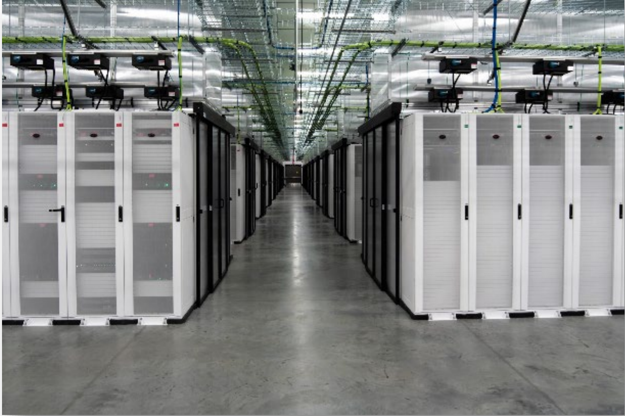
Data Hall with Server Racks (modern style with utilities hung from the roof)
